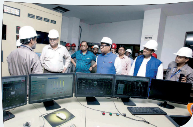
Hon'ble State Minister for Power, Energy and Mineral Resources Mr. Nasrul Hamid MP talking to the officers at the control room during his visit to Barapukuria Power Plant
