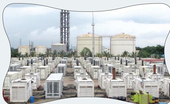
Daudkandi 200 MW Power Plant
