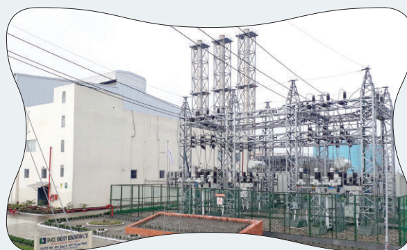
Kamalaghat, Munshiganj 54 MW Power Plant
