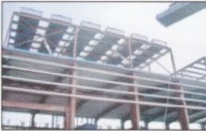
Khulna (KPCL) 115 MW Quick Rental Power Plant Expected Commissioning Date : March, 2011
