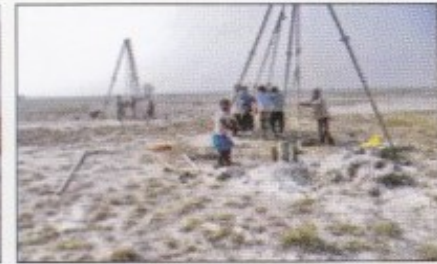
Sirajganj 150 MW Power Plant (NWPGL). Expected Commissioning Date : June, 2012
