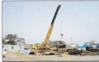
Sylhet 150 MW Peaking Power Plant. Expected Commissioning Date : February, 2012
