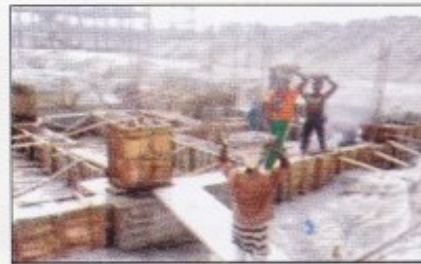
Chandpur 150 MW Peaking Power Plant. Expected Commissioning Date : March, 2012
