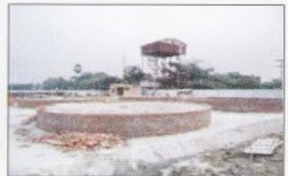
Amnura (Sinha Power) 50 MW Quick Rental Power Plant Expected Commissioning Date : April, 2011
