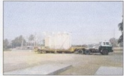
B-Baria 70 MW (Aggreko) Quick Rental Power Plant Expected Commissioning Date : February, 2011
