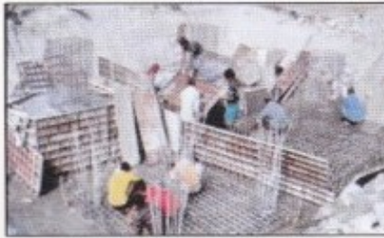
Gopalganj 100 MW Peaking Power Plant. Expected Commissioning Date : August, 2011
