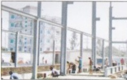
Ashuganj 50 MW Power Plant (TSK) Expected Commissioning Date : April, 2011
