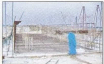
Keraniganj (Power Pac) 100 MW Quick Rental Power Plant Expected Commissioning Date : April, 2011
