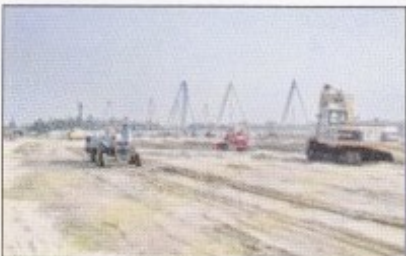
Jaldha, Kamaphuli (Acorn Infra Ser. Ltd.) 100 MW Quick Rental Power Plant. Expected Commissioning Date : April, 2011
