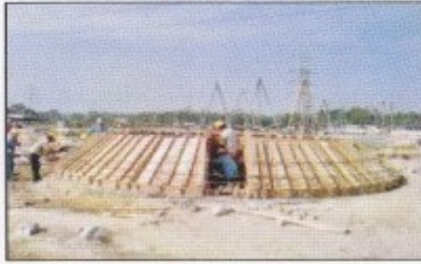
Hathazari 100 MW Peaking Power Plant. Expected Commissioning Date : September, 2011
