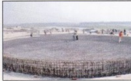
Baghabari 50 MW Peaking Power Plant. Expected Commissioning Date : September, 2011
