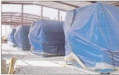
Meghnaghat (IEL) 100 MW Quick Rental Power Plant Expected Commissioning Date : March, 2011
