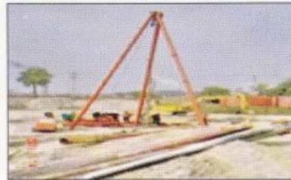
Gazipur 50 MW Power Plant. Expected Commissioning Date : November, 2011
