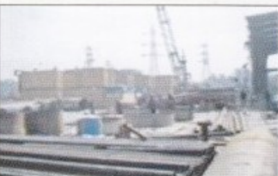
Noapara (Khan Janhan Ali) 40 MW Quick Rental Power Plant. Expected Commissioning Date : April, 2011
