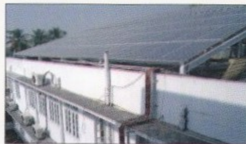
Solar panel at Prime Minister's Office
