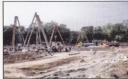
Dohazari 100 MW Peaking Power Plant. Expected Commissioning Date : September, 2011
