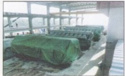
Noapara 105 MW Rental Power Plant Expected Commissioning Date : March, 2011
