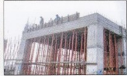
Bera 70 MW Peaking Power Plant. Expected Commissioning Date : October, 2011
