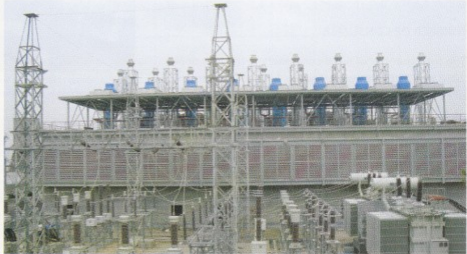
Ashuganj 55 MW Rental Power Plant & Sub-station
