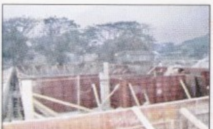
Siddhirganj (Dutch Bangla Power) 100 MW Quick Rental Power Plant. Expected Commissioning Date : April, 2011
