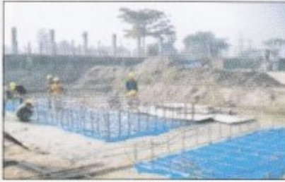
Ghorashal (Max Power) 78 MW Quick Rental Power Plant Expected Commissioning Date : February, 2011
